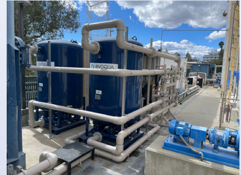
Ion exchange (IX) effectively removes PFAS from groundwater. IX is already in place at three NASA-funded groundwater treatment plants.
