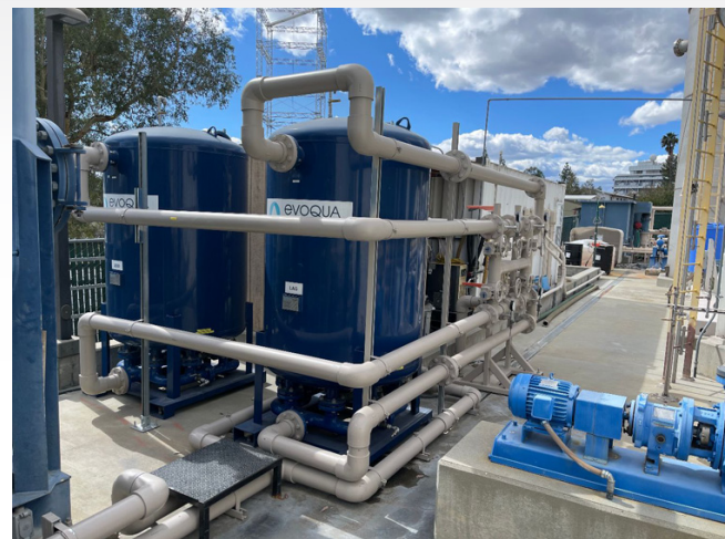
NASA's OU1 source area groundwater treatment system at JPL.
