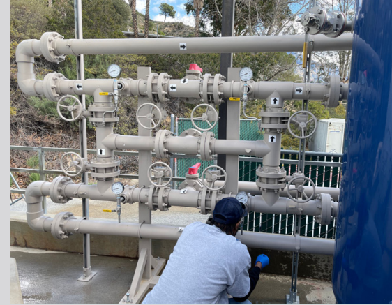
Ion exchange vessels and associated piping removes perchlorate from extracted groundwater.
